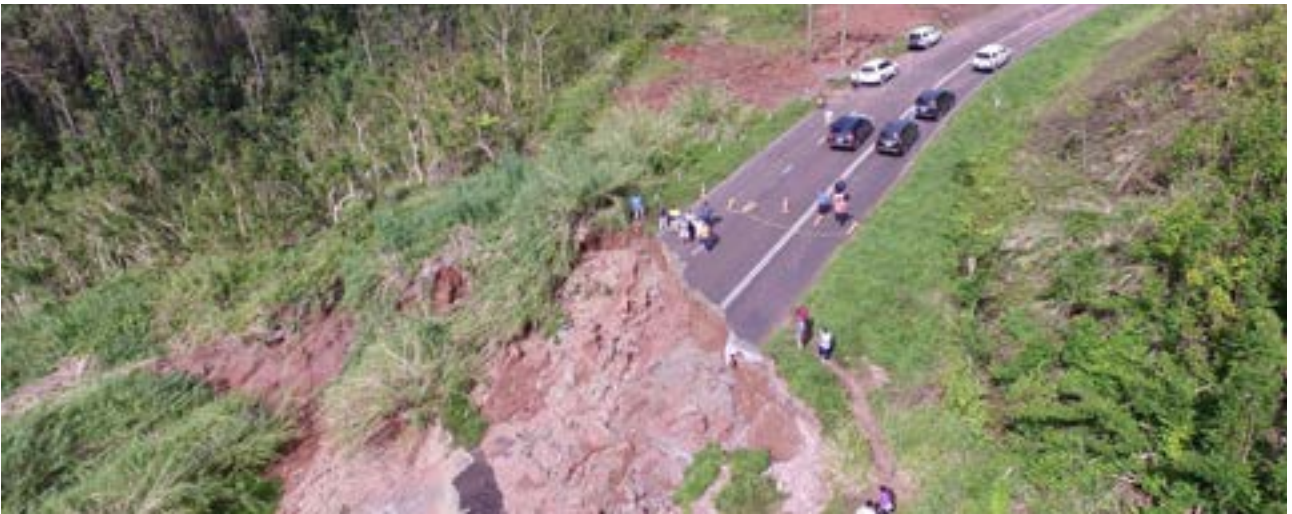
Fig 2. Major landslide in the Northern Division.
